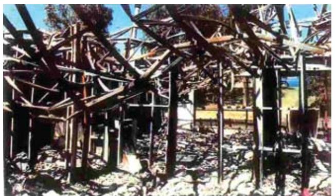
The steel roof trusses have sagged and lost virtually all strength after exposure to the heat of the fire, but the timber-framed stud walls still have sufficient strength to stop total collapse.
