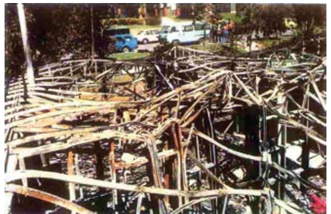
This tangled mess of buckled framing is what remains of a steel-framed house after a fire in the Adelaide area.
